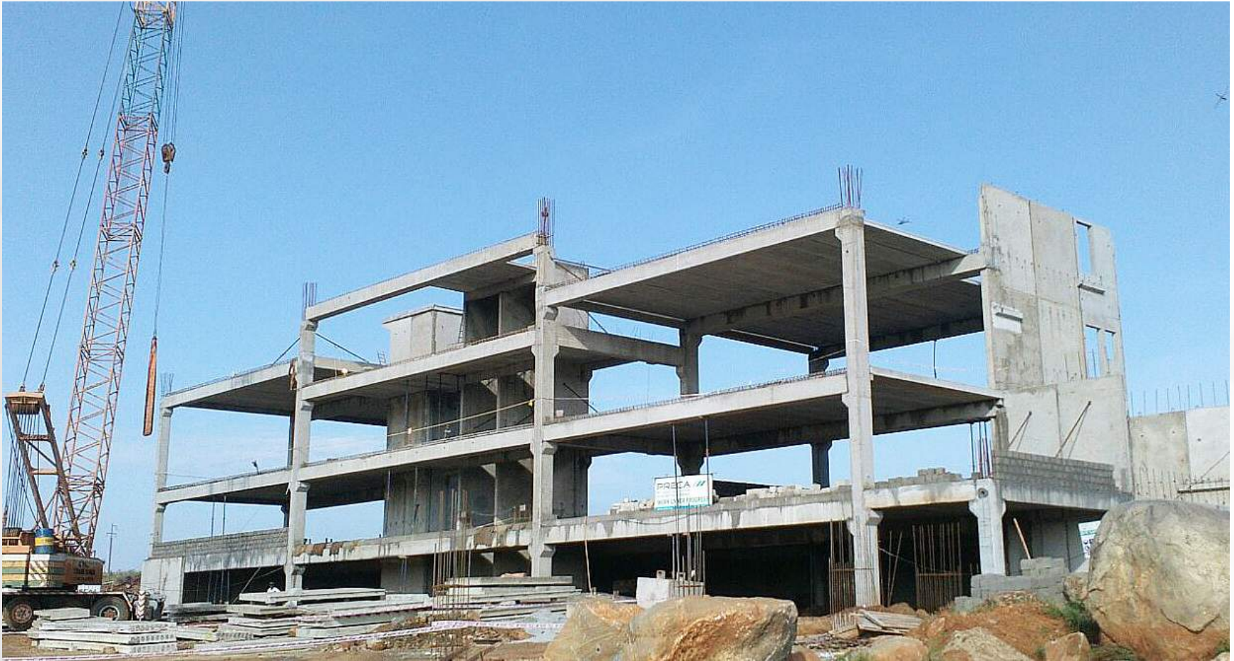
A view showing the progress erection of elements at the Second Floor, the First mostly complete
