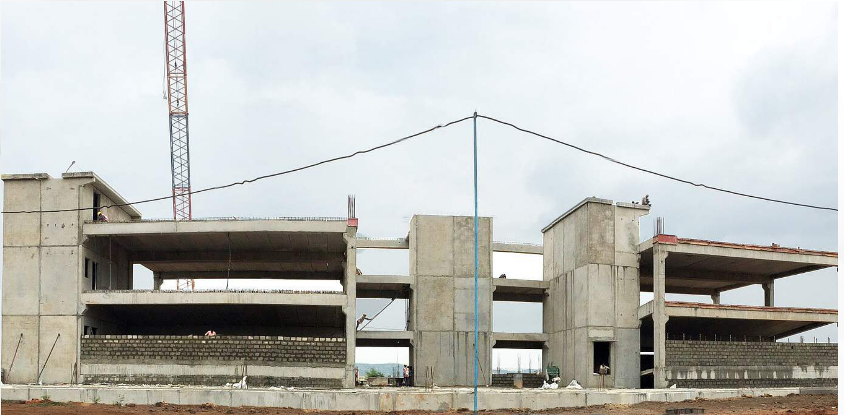
The back view of the Medical Block in the final stages of its completion
