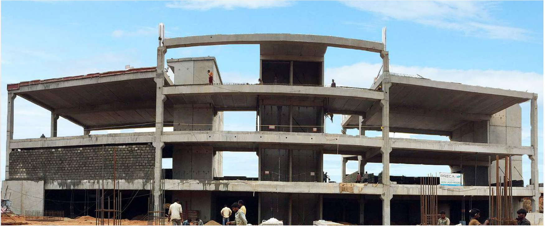
The front view of the Medical Block in the final stages of its completion
