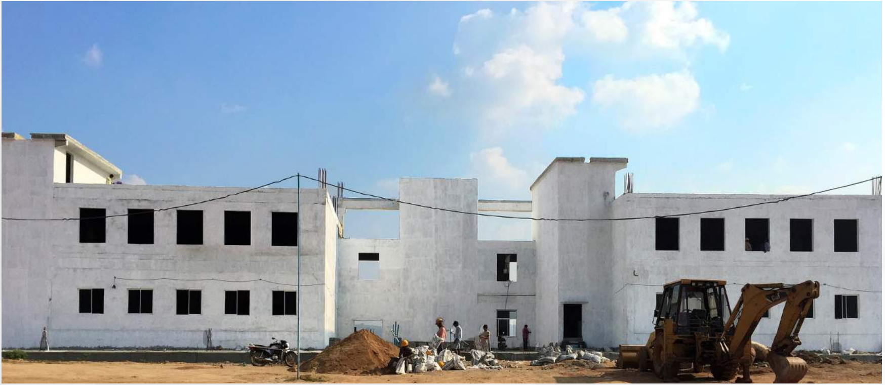
The Medical Block as it sets up to be opened, with the conclusion of PRECA's works
